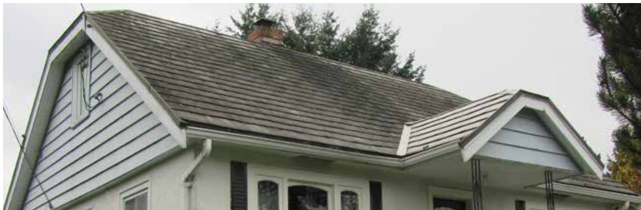
Top left: Existing roof shingles Top right: Brick chimney Bottom: Jerkinhead roof
