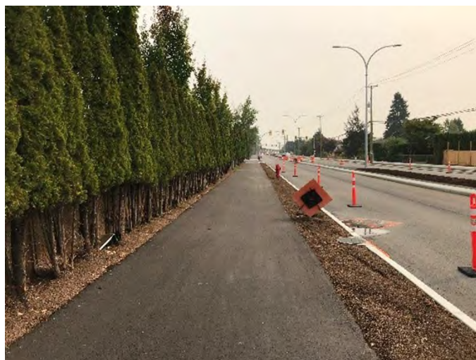
Multi Use Path on 64th Avenue Arterial widening from 184th Street to Fraser Highway.
