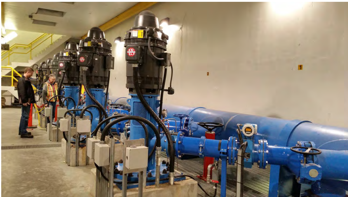
Clayton Drinking Water Pump Station
