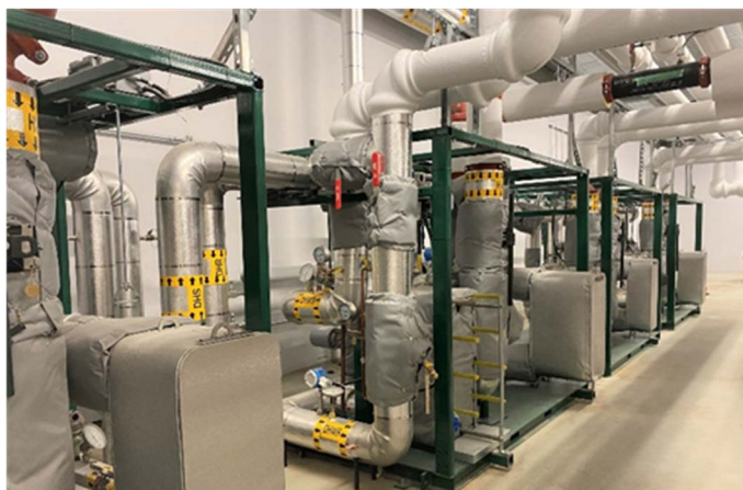
An Energy Transfer Station (the point of delivery for district energy customers) inside of a multi-tower development
