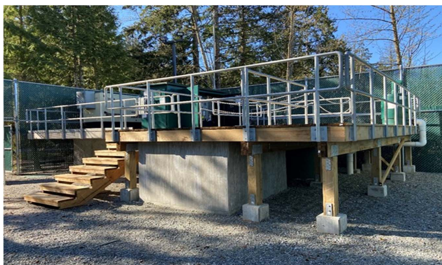
Stewart Farm Sanitary Pump Station Constructed Above Ground Level for Flood Resilience
