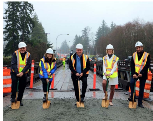
Widening of road made along King George Boulevard Road for the Nicomekl River Bridge Replacement project
