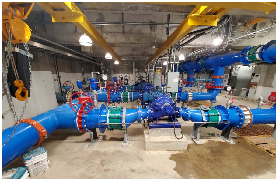
Drinking Water Pump Station
