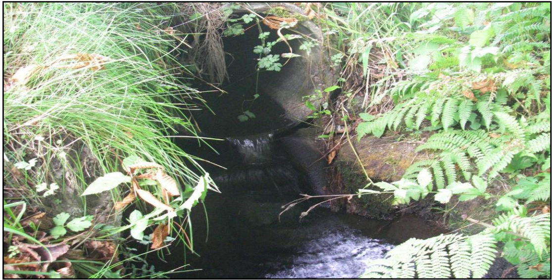
Photo 6. Outflow of second culvert under 96 th Avenue on the reclassified Class A Leoran brook drainage. This culvert (at the very least) likely impedes upstream movement of fish and may limit access to potential fish habitat located on the southern side of 96 th Avenue.
