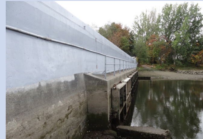
Maintain flood infrastructure: sea dams
