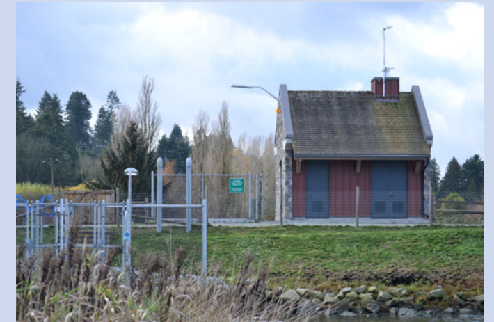
Maintain flood infrastructure: pump stations
