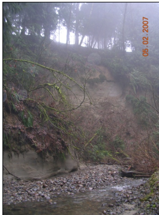
Photo 1: Large Slope Erosion with Houses near Slope Crest, an Example of Undercutting and Slab Regression.
