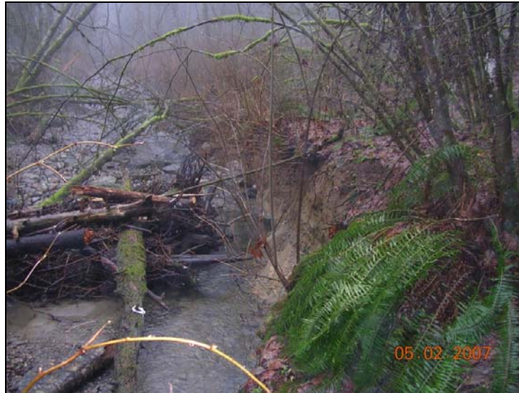
Photo 5: Erosion into Terrace on Right Bank
