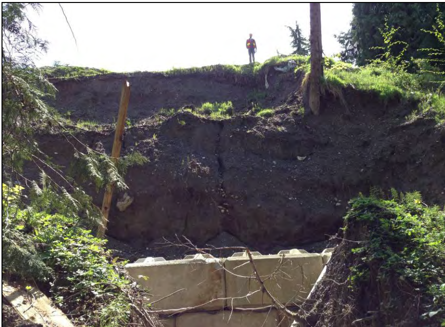
Photo 6: Slope failure risk from steeply excavated fill and native soil with evident erosion.
