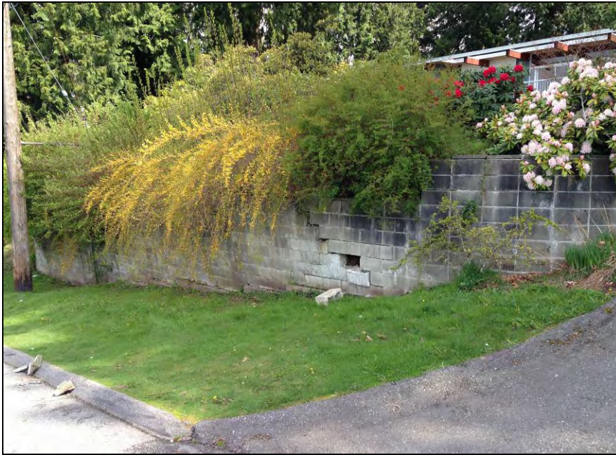
Photo 3: Retaining wall failure along 125B Street.
